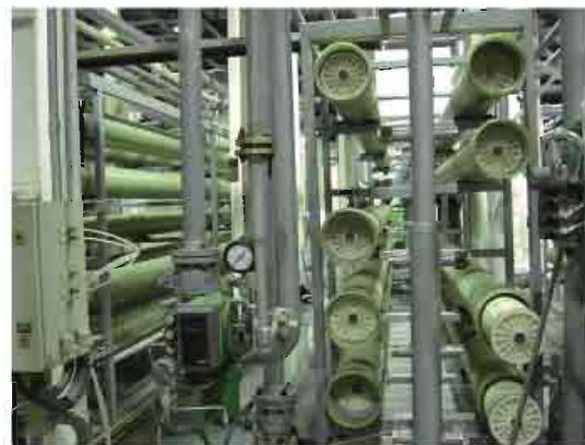
Low-pressure Filtration System
